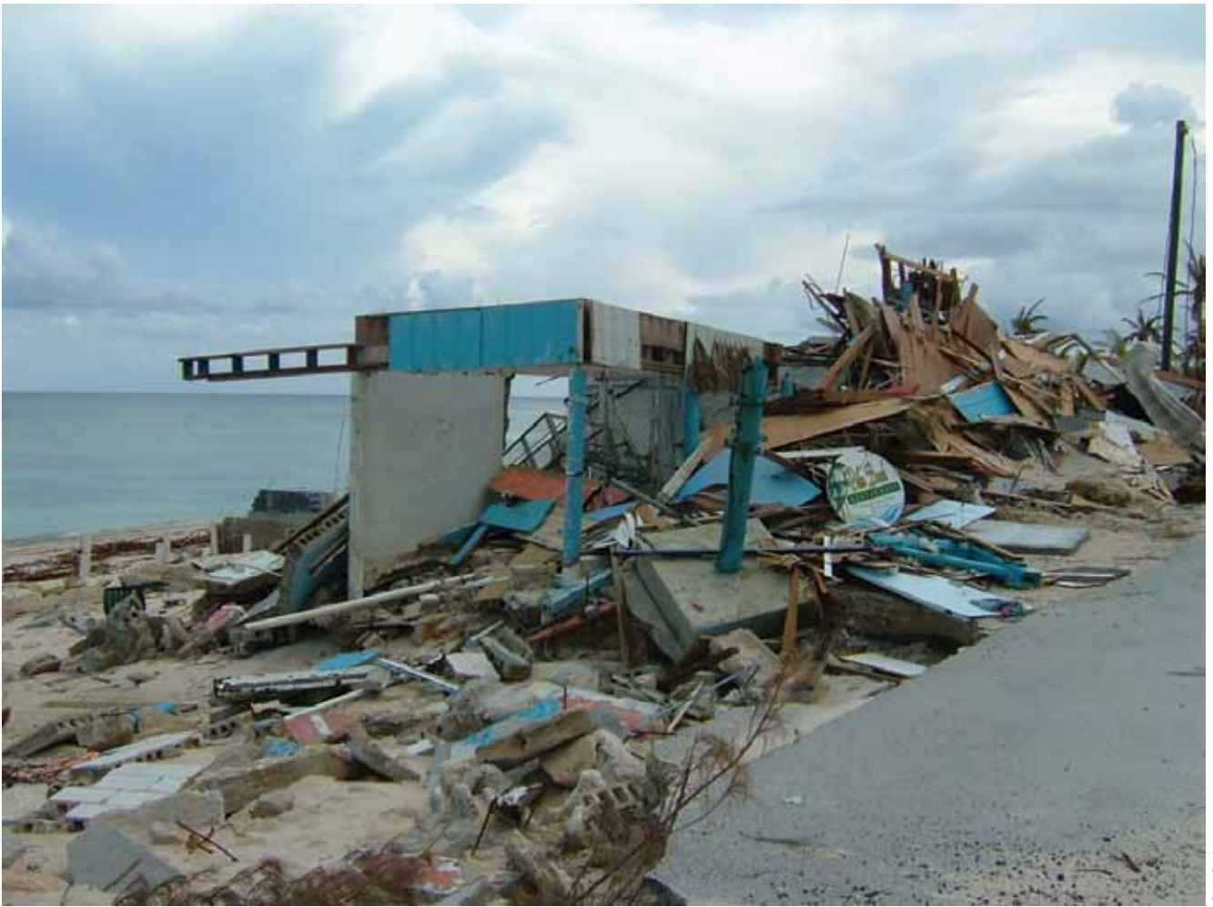
Impacts of Hurricane Ivan on infrastructures in Cayman Islands
